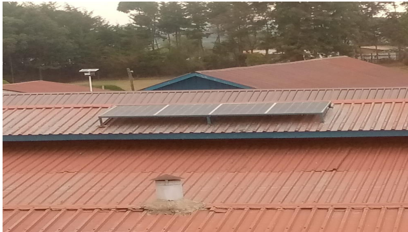
Fig. 1. Photograph of the installed PV Array on the institution's social/ dining hall roof
